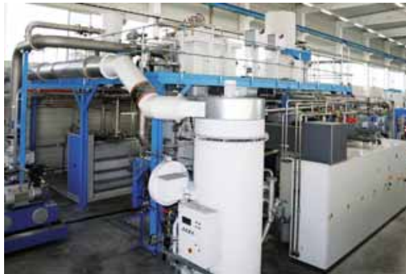
Fig. 3 View of the FCT pilot plant stations with high-temperature furnaces, designed for the combi-process
